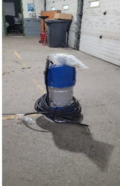
New Pump at the Industrial Park Pond.
