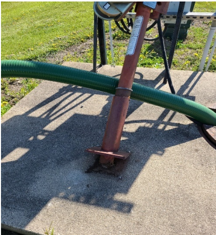
(Damage to pump)
