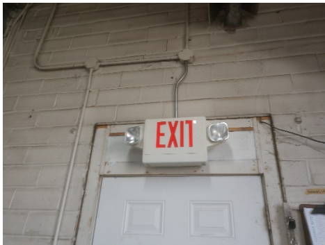
Installed lighted exit sign.
