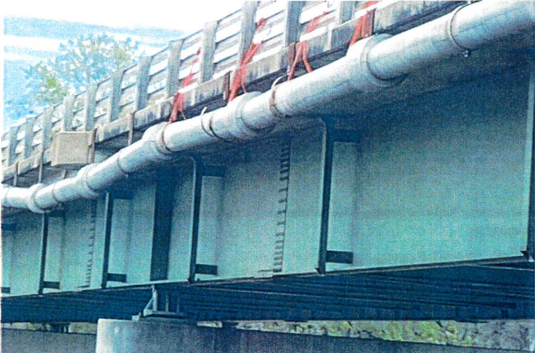
Sanitary Sewer Force Main with Broken Hanger Straps
